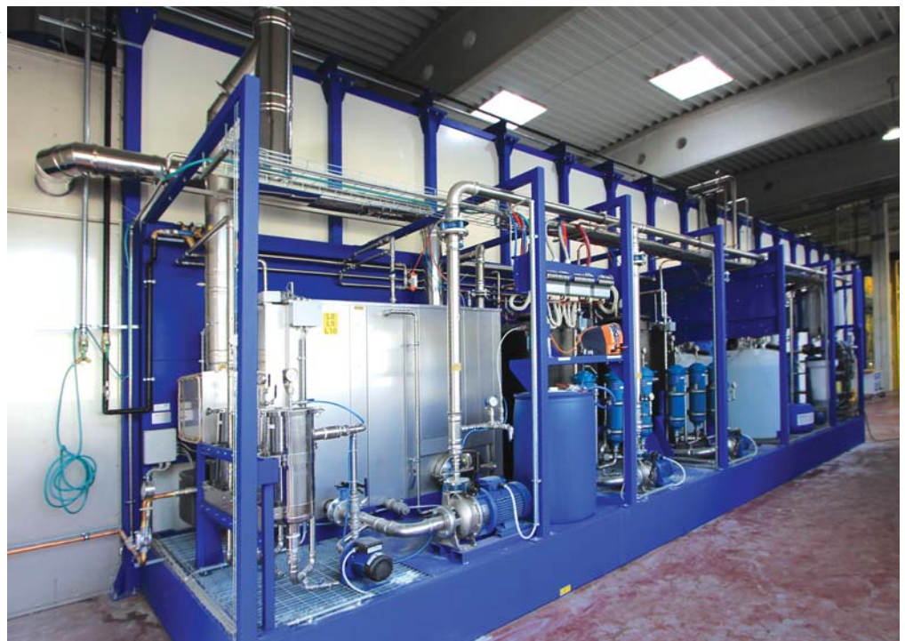
The waste water recovery and filtration skid.
