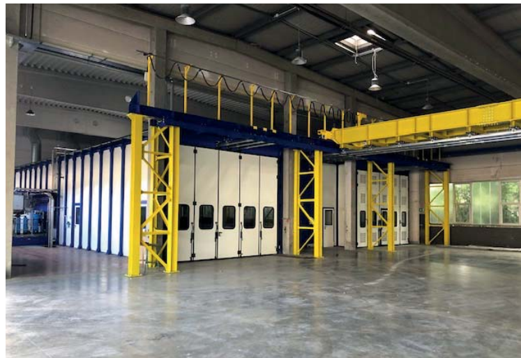
The new plant installed by Eurotherm Spa.
