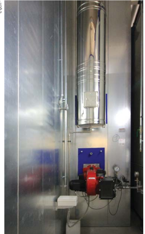
One of two burners with which the curing oven is equipped.
